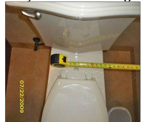
W/C too close to wall and lavatory
