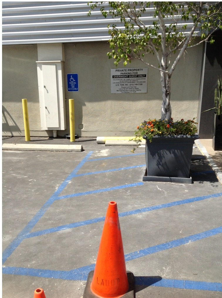
Inconsiderate Placement of Tree Blocks Parking Access Aisle
