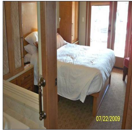
No wheelchair turning space
