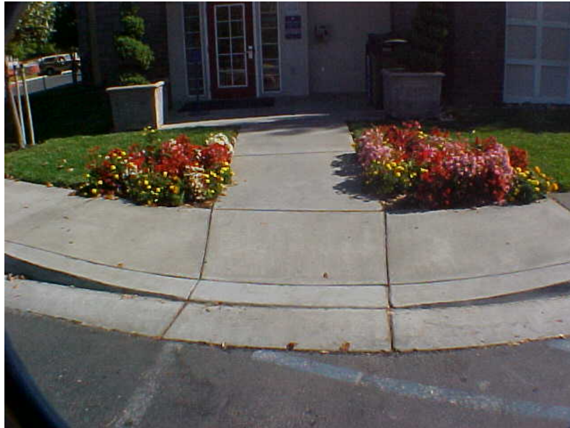
Non-compliant Steep Walkway to Hotel Entrance
