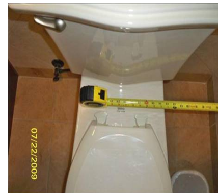
W/C too close to wall and lavatory
